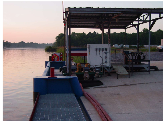
Pumping station near the bulkhead.
